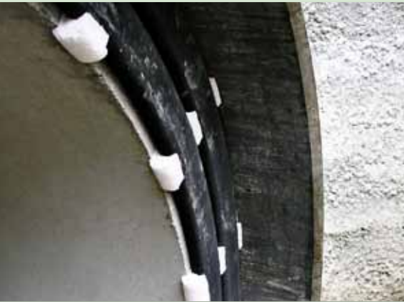
Close-up picture of Hydraulic Joint
