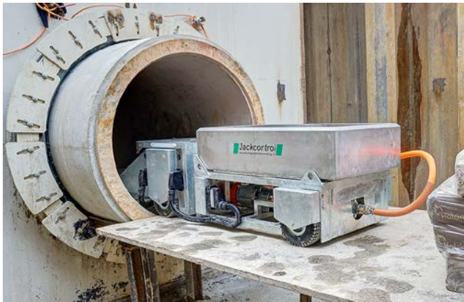
CT ROVER WITH CEMENT TANK/MIXER AND INJECTION PUMP AT THE TUNNEL ENTRANCE
