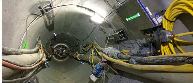
MT.CONNECT MSS BOX INSTALLED IN THE TUNNEL
