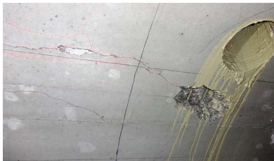
PIPE DAMAGE EXPERTISE
