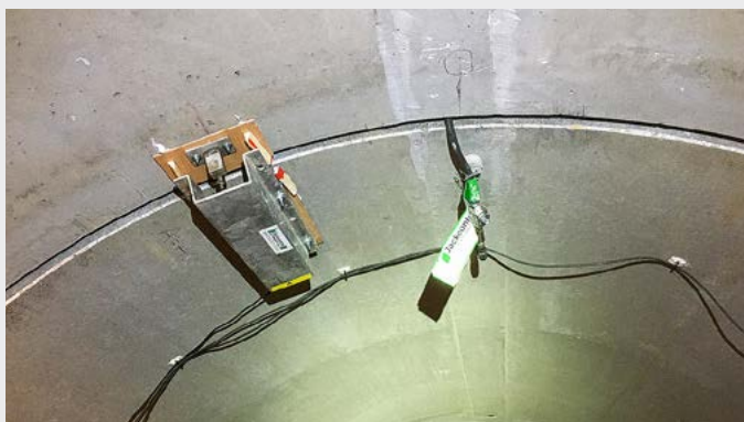
DISPLACEMENT SENSOR IN THE CROWN FIXED WITH GLUE
