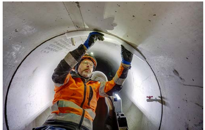
INSERTION OF THE SHUTTERING STRIP INTO THE CAVITY AREA IN PIPE DN 1200 MM
