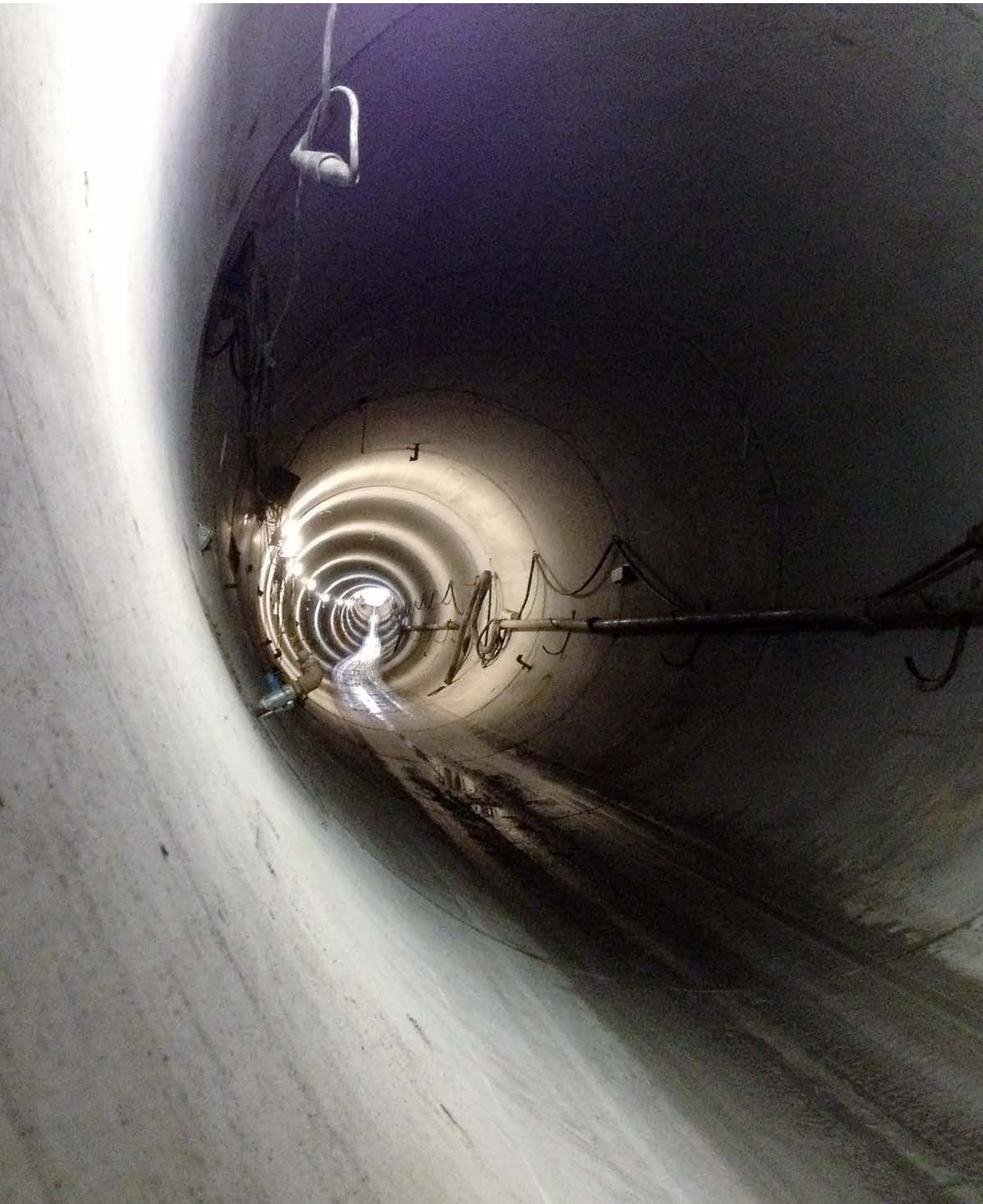
CURVED MICROTUNNEL FOR HYDROPOWER PLANT (SWITZERLAND): R=260 M (PIPE ID 3200 MM, L=3 M)
