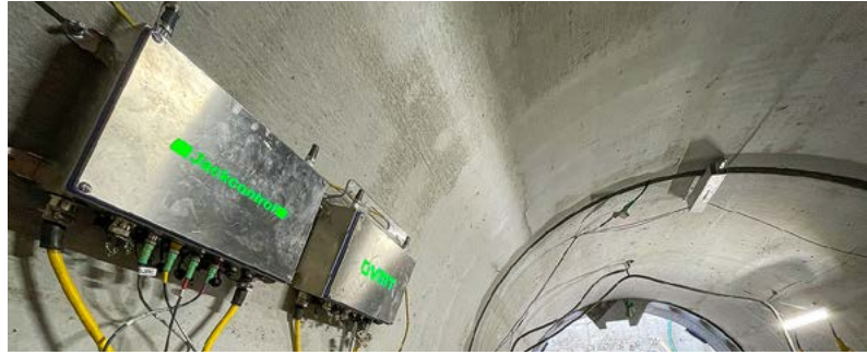
MT.CONNECT BRINGS THE INTERNET INTO THE TUNNEL
